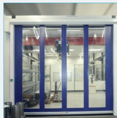
Separation of pre-tempering zone by partition and high-speed PVC gate
